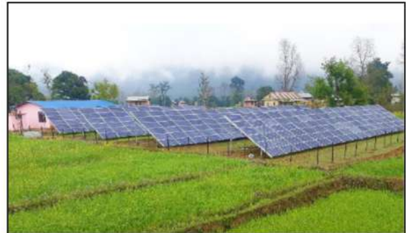
Figure 7: Powerhouse and 100kWp PV array
